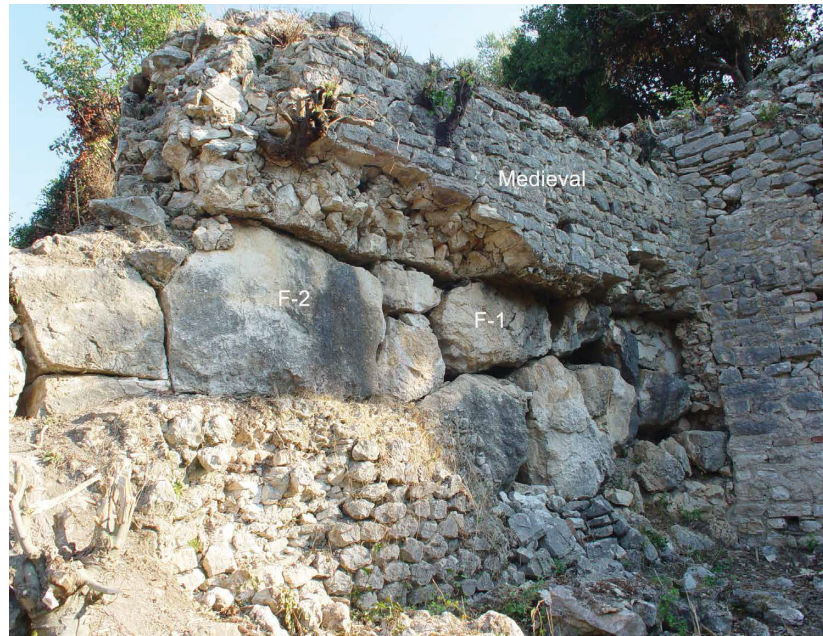
Figure 33. Walls F-1 and F-2, below the medieval fortifications on the Acropolis. D. Hernandez, after photo M. Smith; courtesy Butrint Foundation
