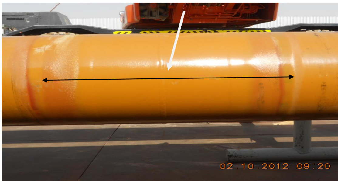
Figure 19—FBE coated Girth Joint area marked within arrow. Girth weld is at center shown by white arrow
